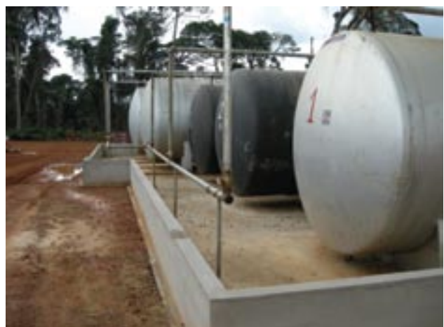
Concrete bunding around major fuel storage tanks at site
